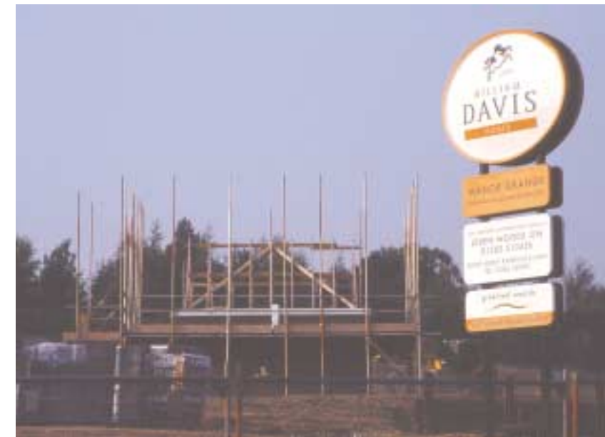
Many developers have landbanks which they hold for many years ahead of building. The long-standing commitment by William Davis Ltd to development in the Brizlingcote Valley has been vital to the success of this project.
